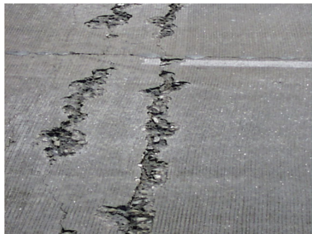
Figure 3. Severe Spalling of CFRCP [11]
