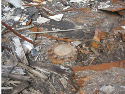
Figure 3. Welded hole in the wellbore SG-3.
