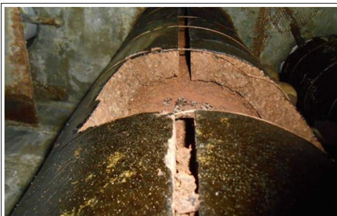
Fig.1. CUI in insulated carbon steel tube
