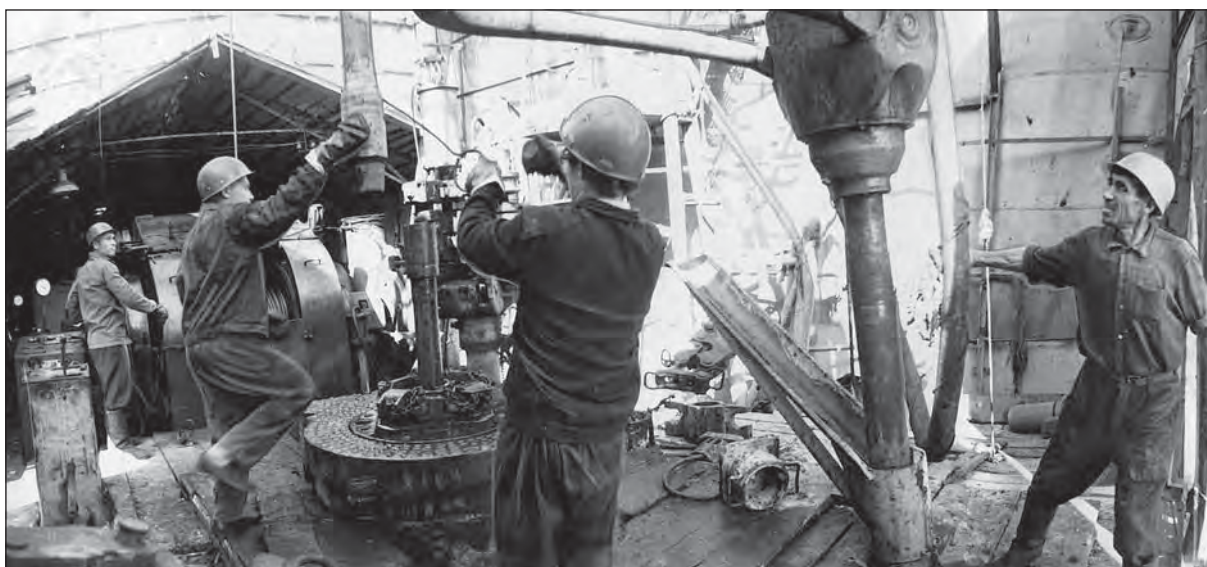
Drilling of the oil well led by M. Grin's best brigade. Aznakaevo drilling department of the 'Tatneft' association. Almetyevsk. 1975. National Archive of the Republic of Tatarstan
