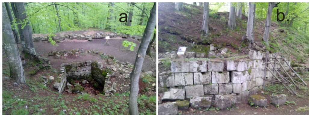
Fig. 5. Structural-functional instability and deterioration of immovable heritage: a. Root wedging affecting the walls from the eastern slope of Dacian Fortress – Sarmisegetusa (a UNESCO World Heritage Site, ID 906-001) from the Orăștie Mountains, Hunedoara County, Romania. b. Basic measures to stop the collapse of the fortress walls
