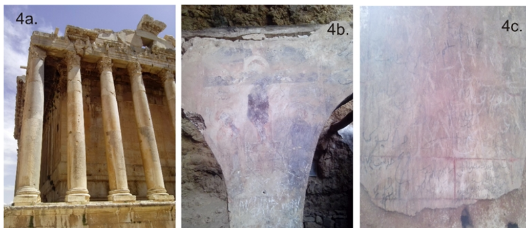
Fig. 4. Structural-functional instability, paintings and writings degradation of immovable heritage: a. Instability of the decorated roof at Temple of Bacchus, part of Baalbek Roman Archaeological Site (the largest and most impressive Roman temple complex in the world, part of UNESCO World Heritage since 1984, Beqaa Valley, North-eastern Lebanon); b. Degradation of Christian paintings from Deir es-Salib, inside the grotto with the same name, Qadisha Valley (The Holy Valley), a UNESCO World Heritage site (ID 850-001), North Lebanon; c. Degradation of three type of writings from Deir es-Salib (Arabic, Greek, and Syriac)
