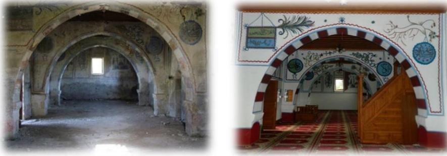
Image 11: Condition of harim (before 2004 restoration)
